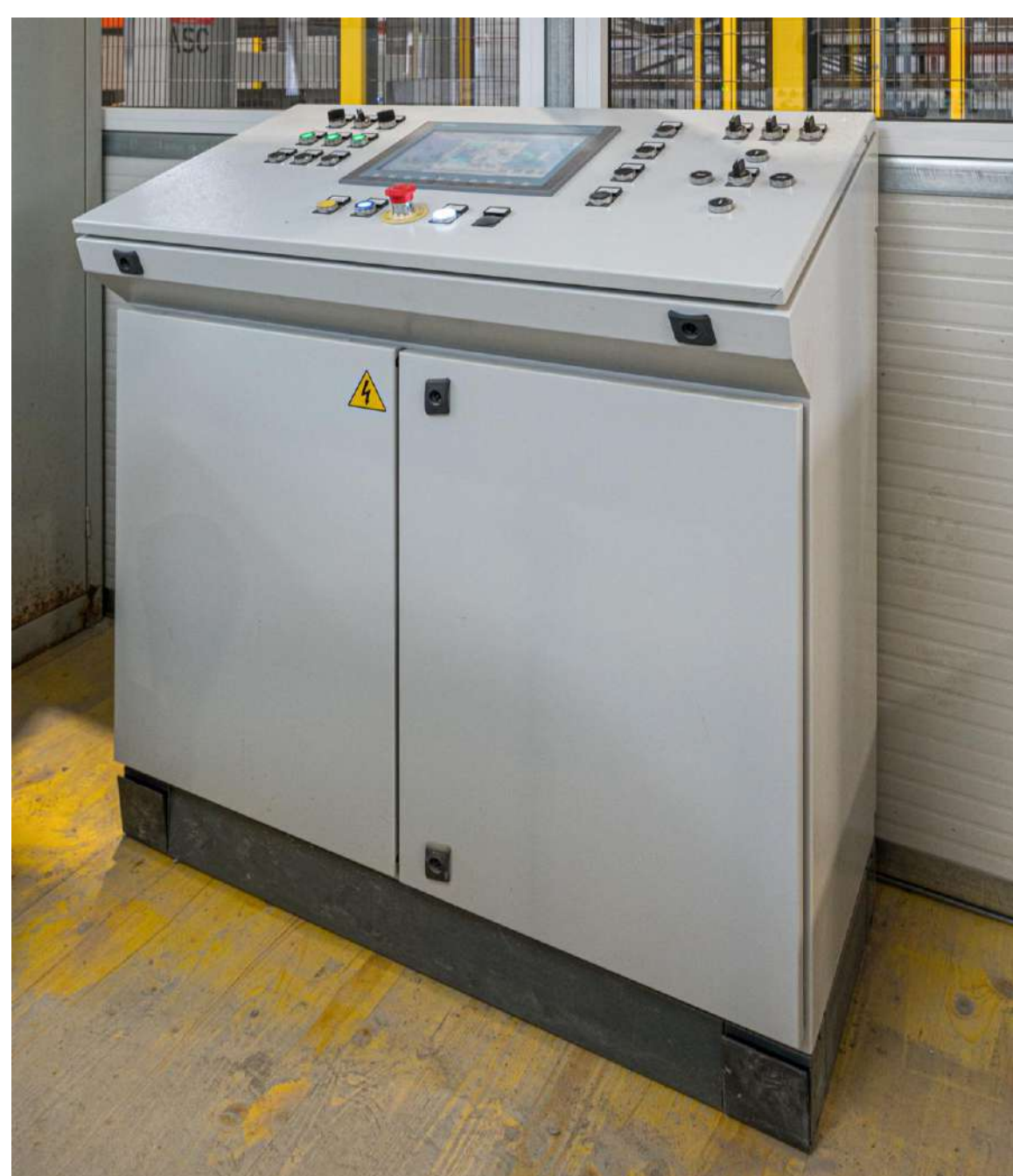
Control Panels and Consoles
